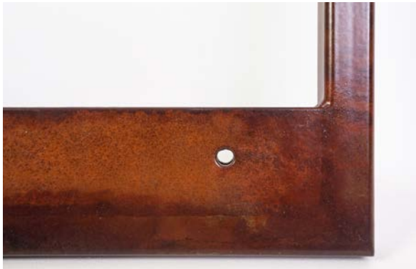
Rusty esthetics naturally rusted steel construction
